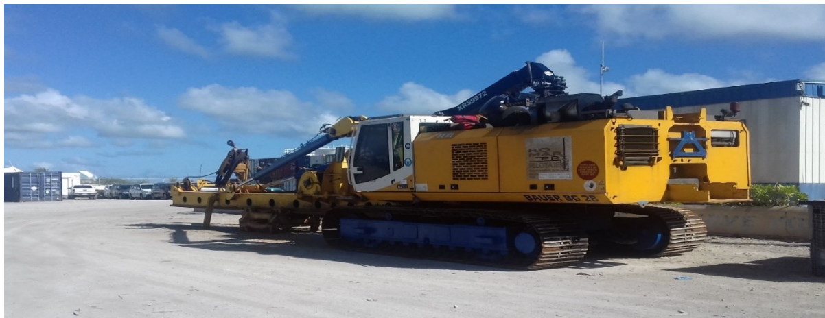
Arrival of Rotary Drill at South Dock, Provo for the Ritz Carlton Project
