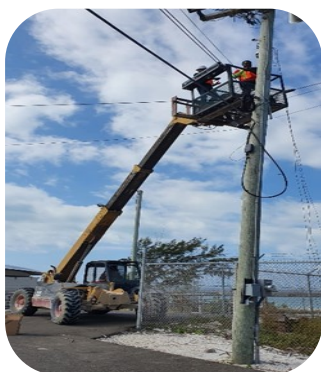
Grand Turk, CCTV Project
